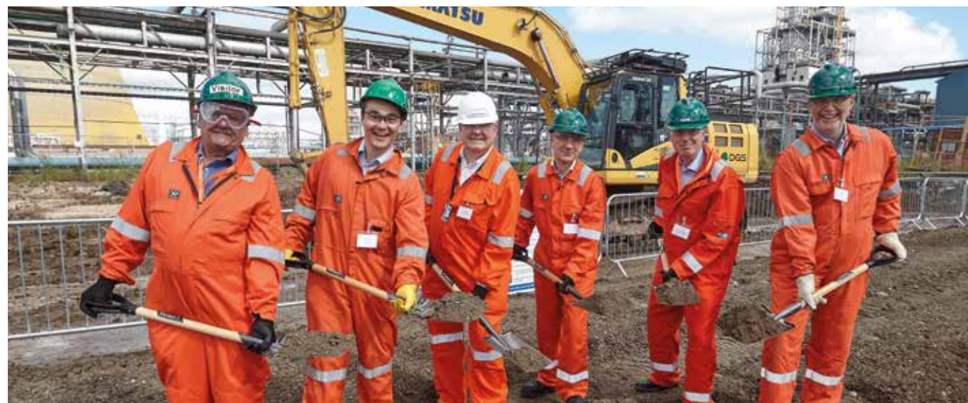
Gerard Britchfield, Coillte COO & CFO (fourth from left), with representatives from the Tricoya Consortium at the breaking ground ceremony for the world's first Tricoya® wood chip acetylation plant at Saltend Chemicals Plant, Hull, UK
